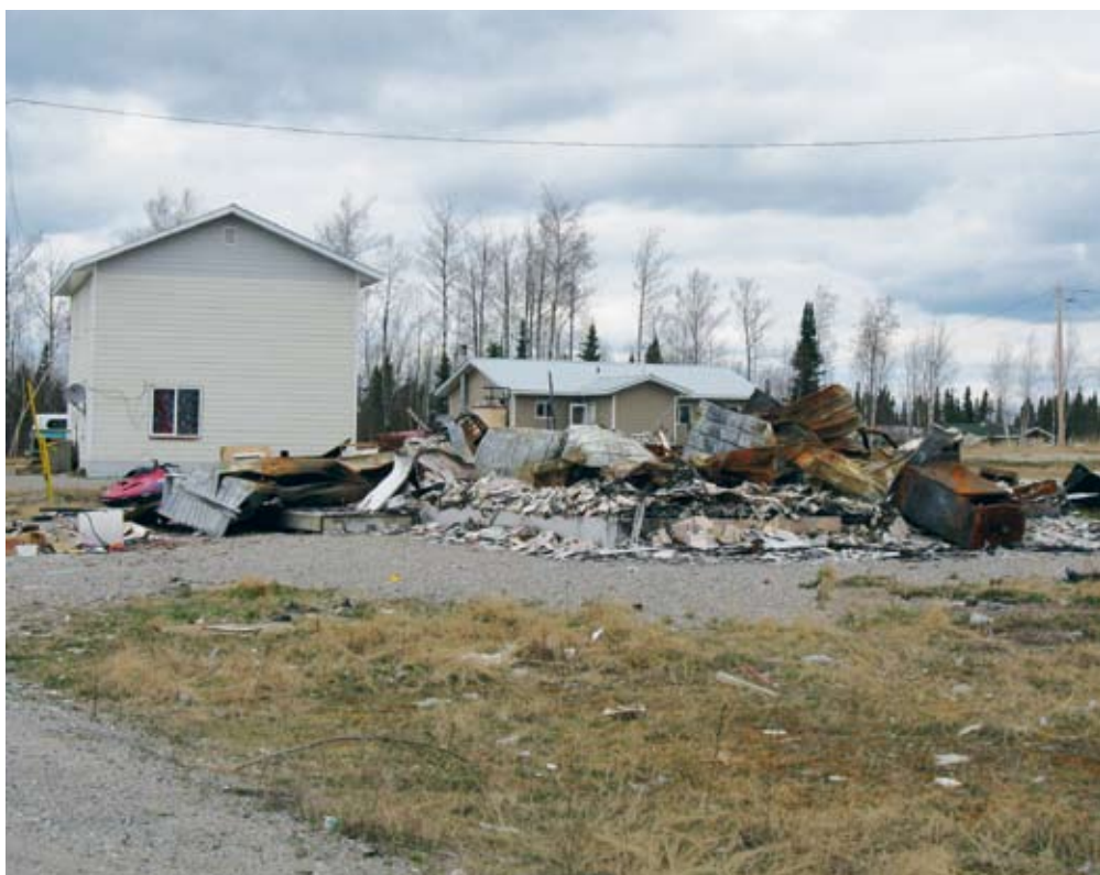
Because of arson, Mishkeegogamang no longer qualifies for insurance on many of its buildings.
