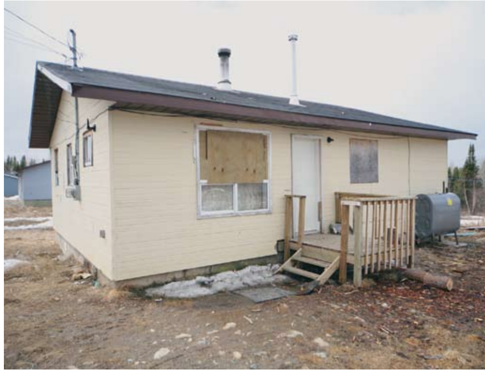
The new renovation program will enable many houses to be upgraded and repaired.
